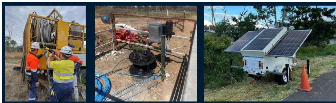
Figure 9. Distributed fibre optics deployment including CSIRO mobile monitoring trailer
